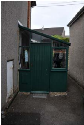
ES05. TIMBER PORCH - TO BE REPLACED
