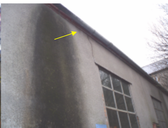
P2 Gaps under barge boards, building 2
