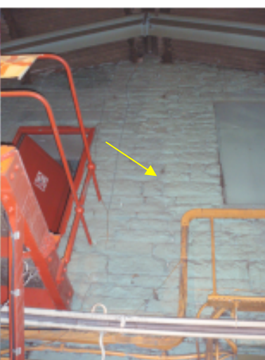
P4 Gaps in masonry, building 3
